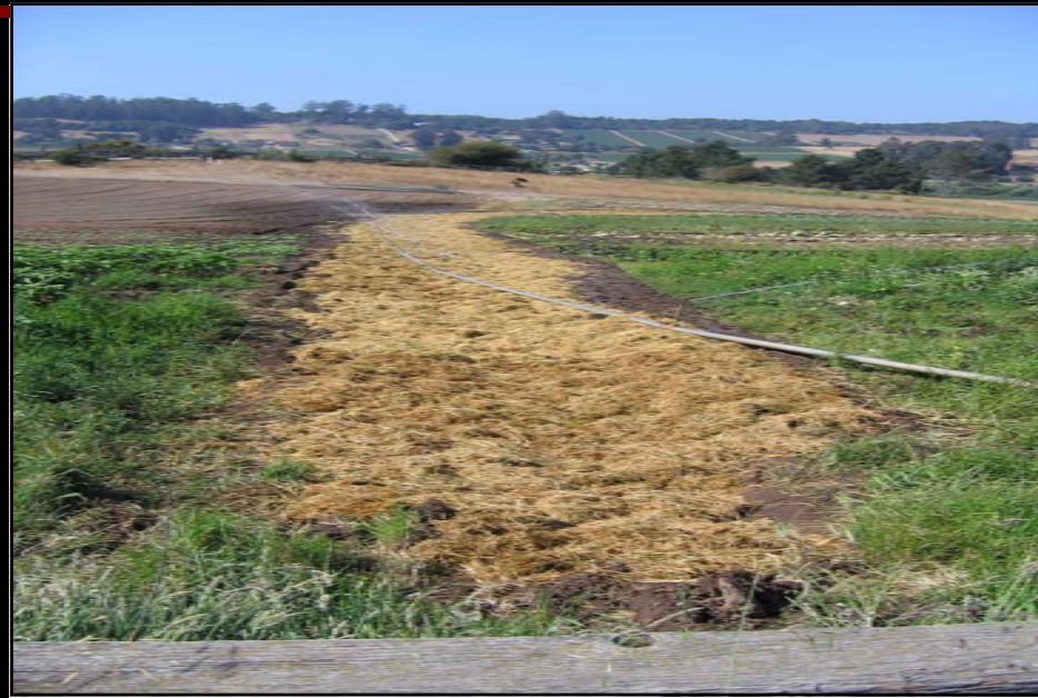
A 500 foot grassed waterway was successfully installed at ALBA's Triple M Ranch in Monterey County.
